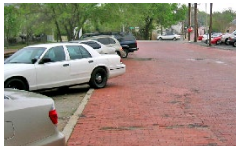
Historic brick streets require special maintenance.
