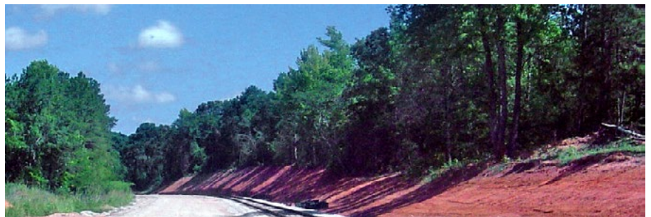
Rail beds no longer in use can become pedestrian and bicycle trails.
